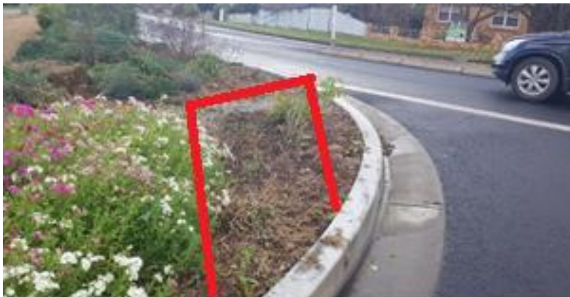
Figure 3 – indication of damage
