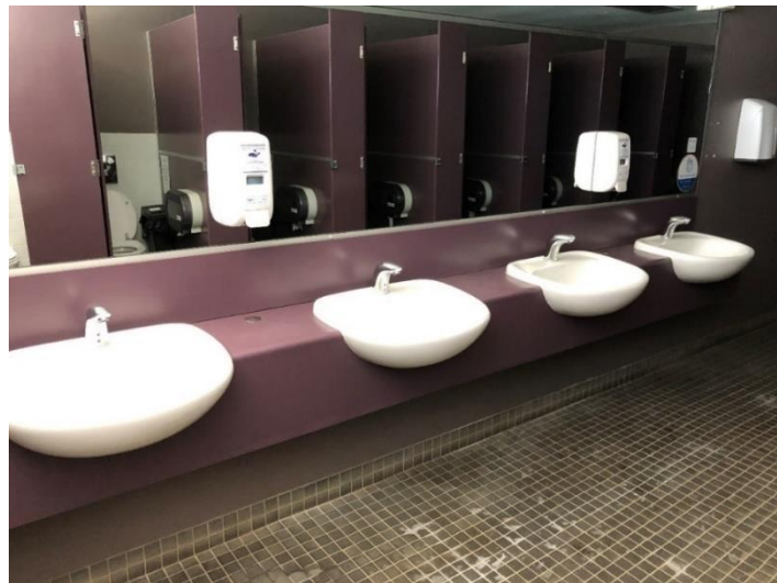
Installation of sensor taps in multiple AELEC bathrooms. This rollout will continue this financial year
